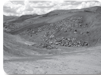
One of many decorative top rock treatments that will be on the I-580 project.
