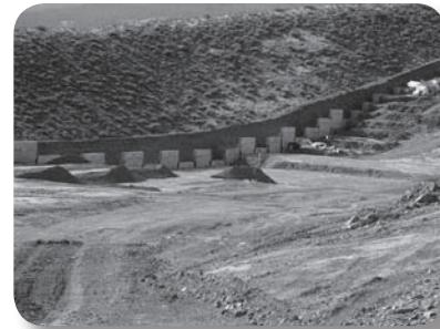
Lower portion of retaining wall under construction between Steamboat Hills and Pleasant Valley Bridges.
