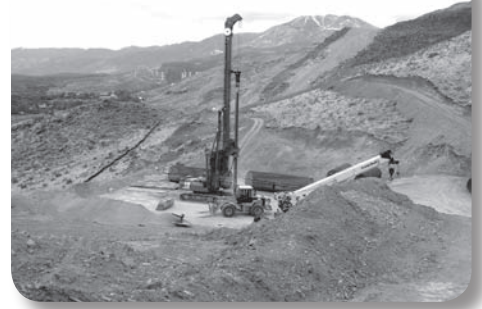
Pleasant Valley Bridge Excavation and drill rig set up for drilling concrete piles for bridge foundation. June 5, 2007
